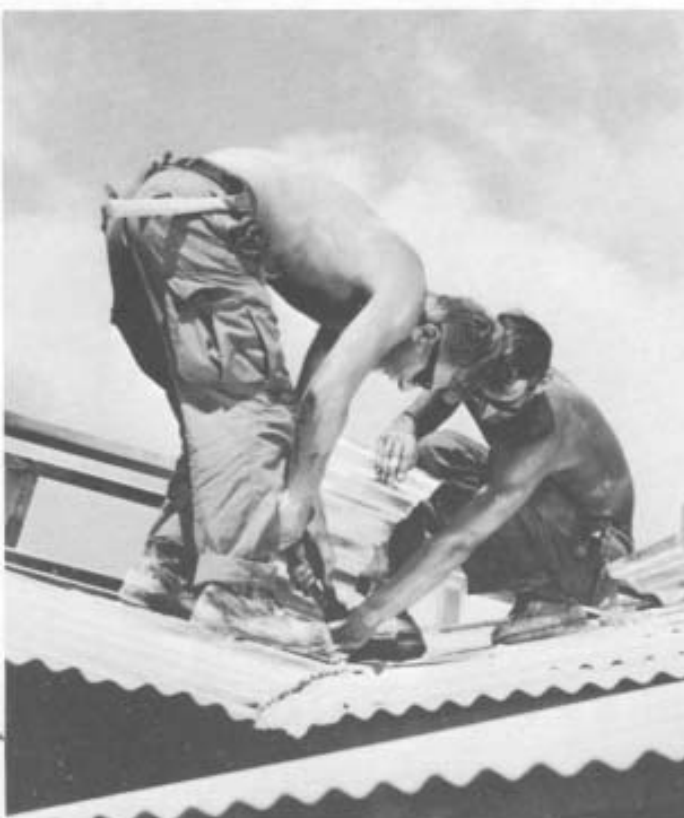
Seabees of Mobile Construction Battalion Seven cover a roof with corrugated tin at Dong Ha.
