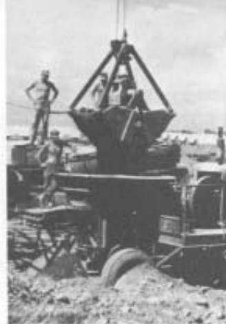
MCB7 Seabees crush rock for cement at Dong Ha (PH1 K.E. Bumpus)
