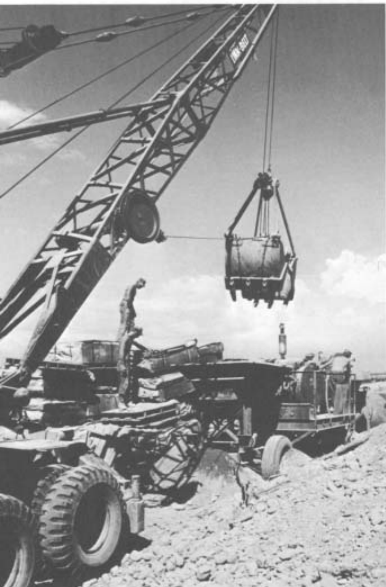
Rock pile grows as Seabees crush rock to use on road construction in South Vietnam. (PH1 K.E. Bumpus)
