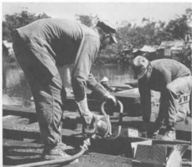
Seabees of MCB 121 cut plank for bridge across the Lang Co River. (PH2 Lucas)
